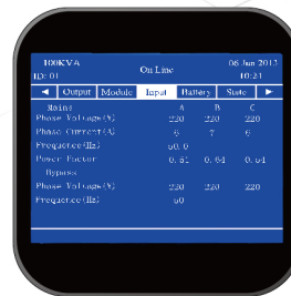
UPS Cabinet Control Panel
